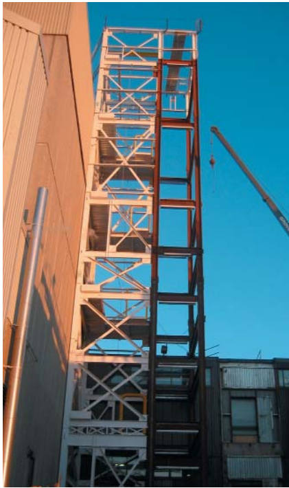
Oland’s new fermenter building stands on its own next to the brewery’s existing foundation.
